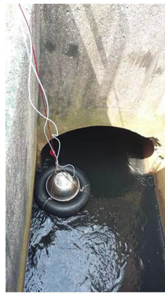
S13 - Settled Sewage Overflow Chamber (SOC)
