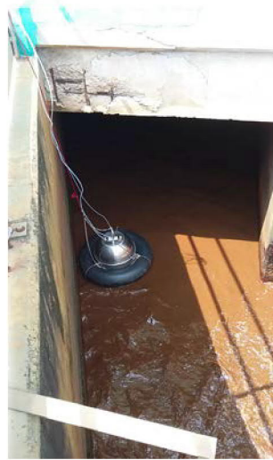
S10 - Return Activated Sludge Screw Pump Pumping Station
