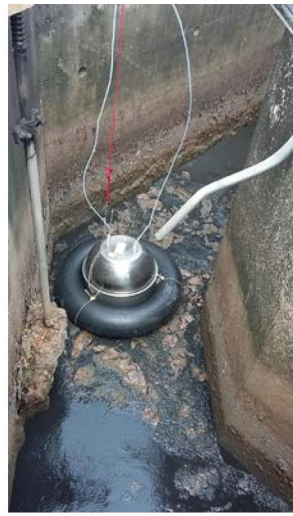
S12 - Primary Sludge Distribution Chamber/Measurement Chamber
