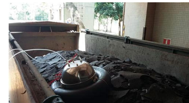
S9 - Dewatered Sludge Skip at Sludge Deratering House
