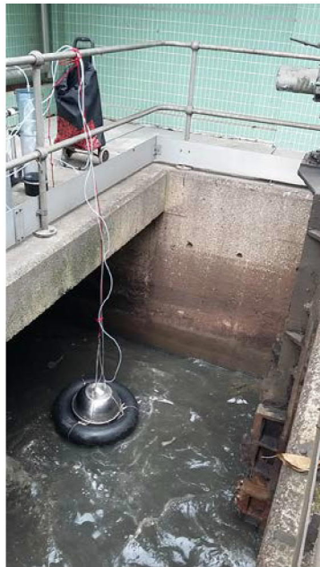
S1 - Screw Pump Pumping Station
